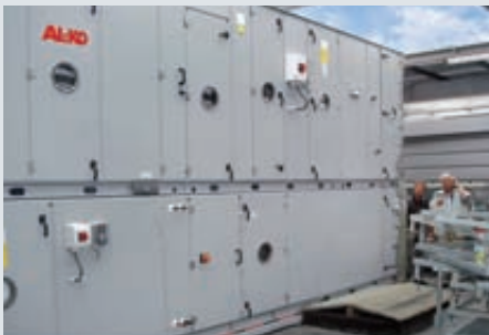
External absorption unit in the accessible roof casings
